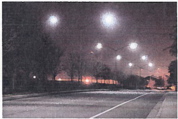
Figure 2: BridgeLux LEDs installed on Las Positas Road
